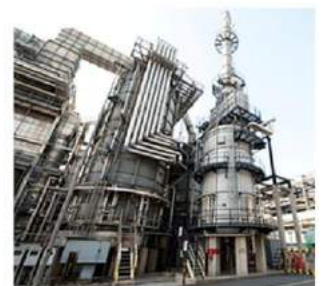
Hydro-treater/HDS Heaters Hydro Cracker Heaters
