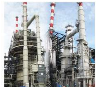
Re-boilers / Hot Oil Heaters
