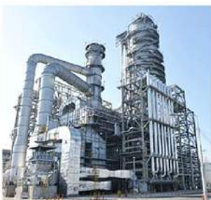
Vacuum Distillation Unit (VDU) Heaters
