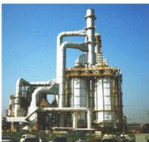
Crude Distillation Unit (CDU) Heaters
